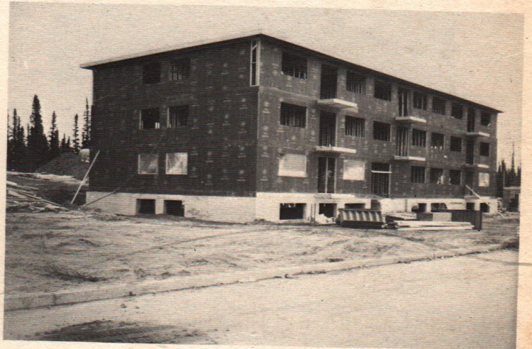
Construction of a privately owned apartment building at Wabush. This block will provide 24 new dwelling units. The construction of another apartment building has also commenced.
