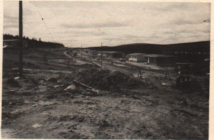
A view of Grenfell Drive in July. Contractors were then busy relocating and installing the hydrants while getting the road beds ready to receive the asphalt.
