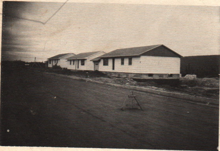
Construction of three houses by the Federal Department of Transport for its Wabush employees. The houses are being built by a local Contractor. They should be ready for occupancy early this fall.
