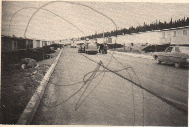
Major work was started in June on the streets of the new Wabush residential area. Street paving is now in progress along with the construction of curbs and sidewalks.
