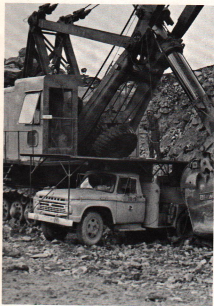
Typical of the innovative spirit of the Griffith's employees is the ingenious scaffolding built by maintenance welders on top of their truck. The platform provides convenient and safe access for servicing equipment like this electric shovel. In cold weather, canvas curtains enclose the rear of the truck, providing a small workshop area protected from the elements. The used tire mounted on the shovel serves as a protective bumper.
